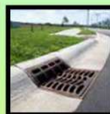
Storm Water Drains
